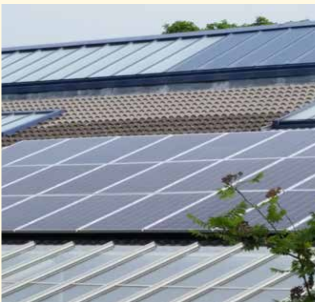
Chilton School, rooftop solar
