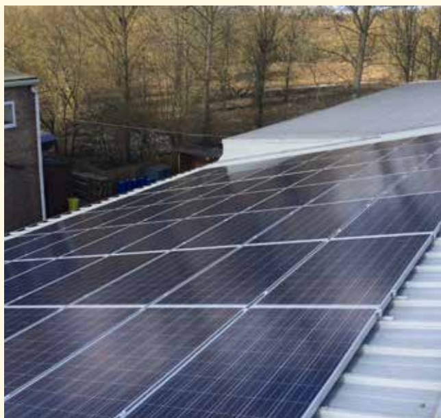
Owen Mumford, rooftop solar
