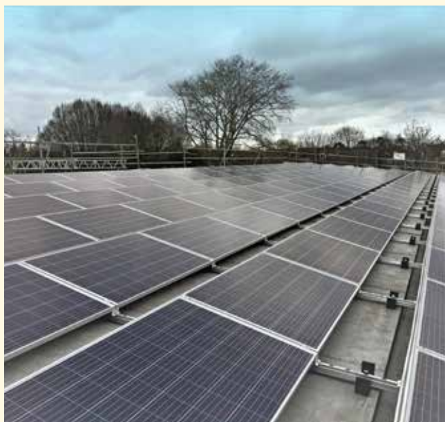
Brookside School, rooftop solar
