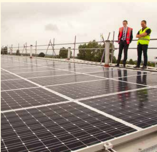
Oxford Bus Company, rooftop solar
