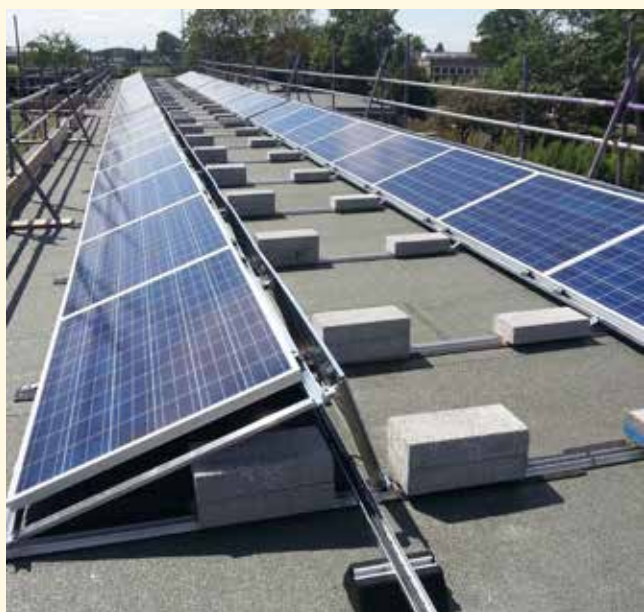
Edward Field Primary School, rooftop solar
