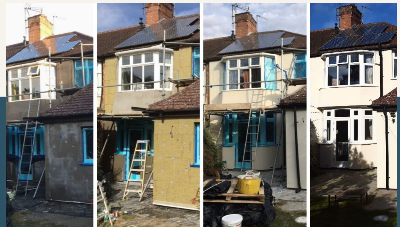
Image 15: Eco-retrofit of an East Oxford terrace through the Cosy Homes Oxfordshire Service, copyright Cosy Homes Oxfordshire
