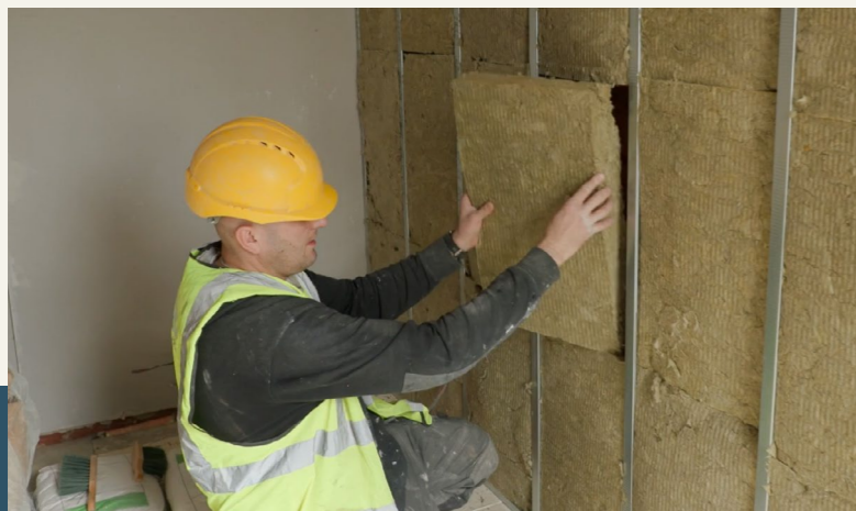
Image 13: Wrapping a house in insulation through the Cosy Homes Oxfordshire Service, copyright Cosy Homes Oxfordshire
