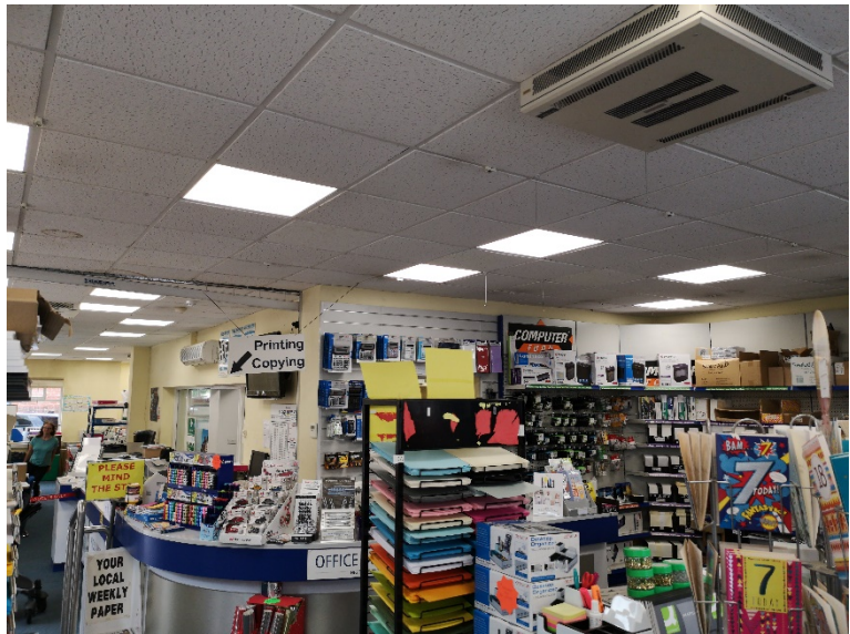
The new lighting in the shop
